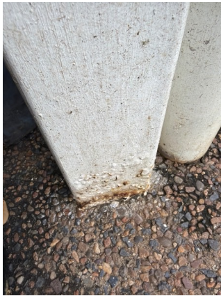
Image of corrosion effecting steel posts.
