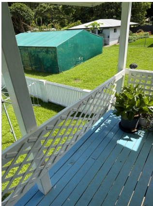
Image of non compliant handrails.
