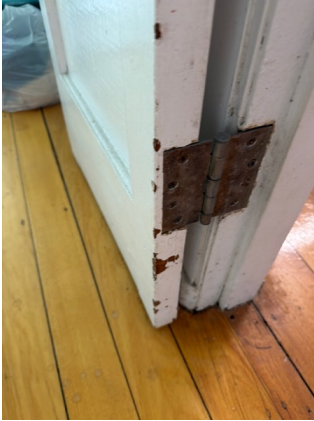
Image of wear and tear to internal doors, consultation with painting professional advised.
