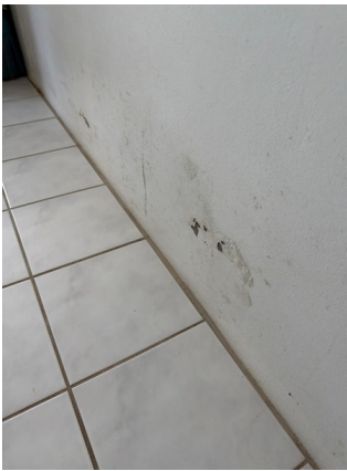
Image of moisture effected sub floor wall.
