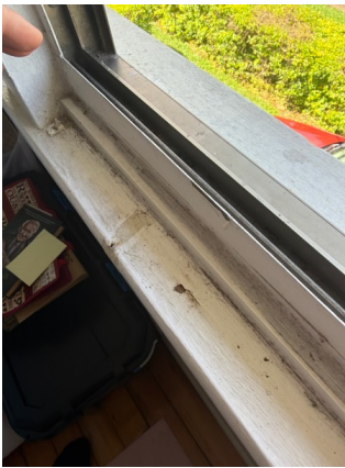
Image damaged window sill timbers.
