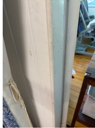
Image of wall wear and tear. Consultation with painting professional advised
