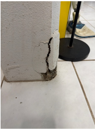
Image of damaged pier.
