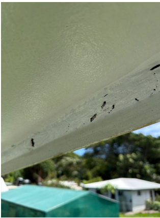
Image of moisture effected eave section.
