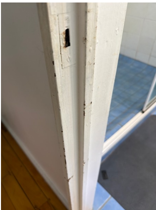
Image of internal door jamb requiring additional protective paint coverings.
