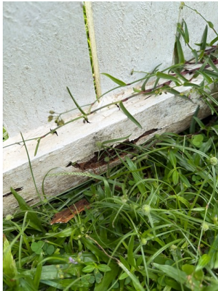
Image of decay effecting fencing Timbers.
