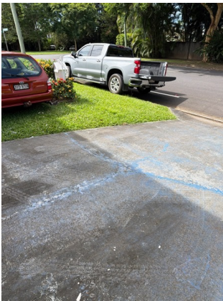
Image of driveway cracking.
