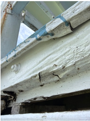
Image of damage to joists.
