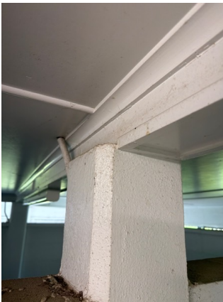
Image of missing ant shields.
