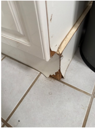
Image of moisture damaged vanity Timbers.
