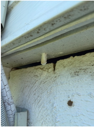
Image of incomplete wall tie down point.
